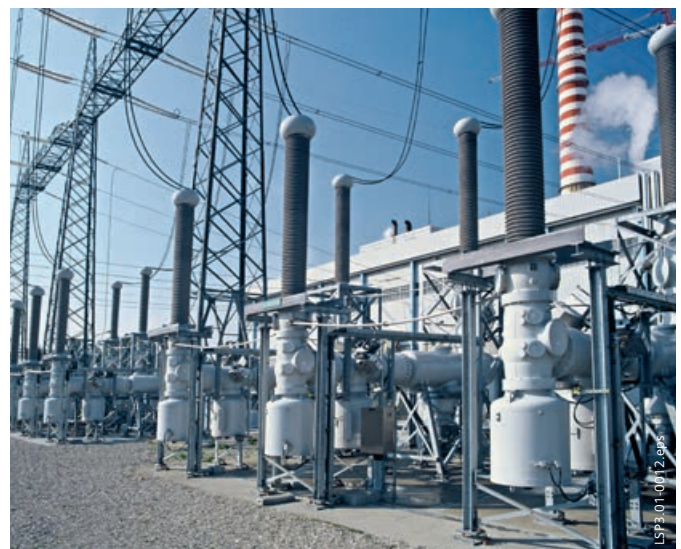
Fig. 1/8 Application in a high-voltage power system
